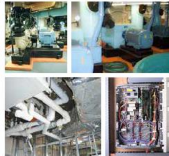
Picture 3: Intelligent Upgrade of Internal System
